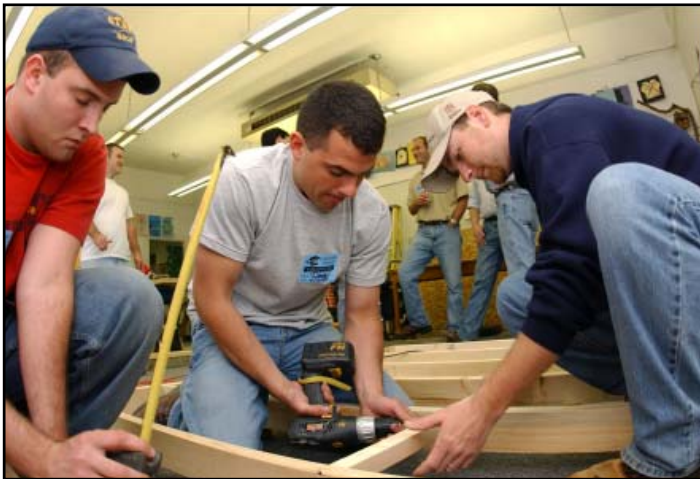
CMA members construct a multipurpose “learning tree house” in a University School fifth grade classroom.
