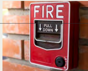
Safety Lighting & Fire Alarm System Phase II $1,600,000
